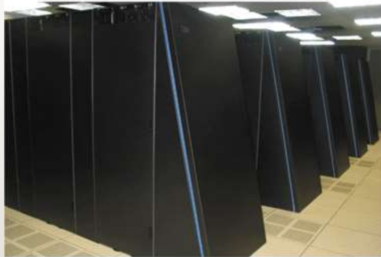
BLUE GENE/L SUPERCOMPUTER This supercomputer is installed at Lawrence Livermore National Laboratory.
